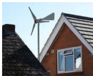
Micro Wind Turbine on a roof top
