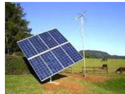
A Wind – Solar PV Hybrid
